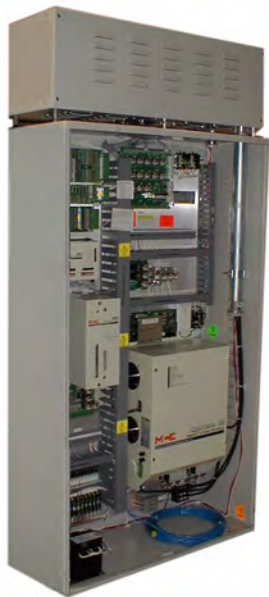
IMC-Performa DC Controller with MCE 12-Pulse SCR Drive
