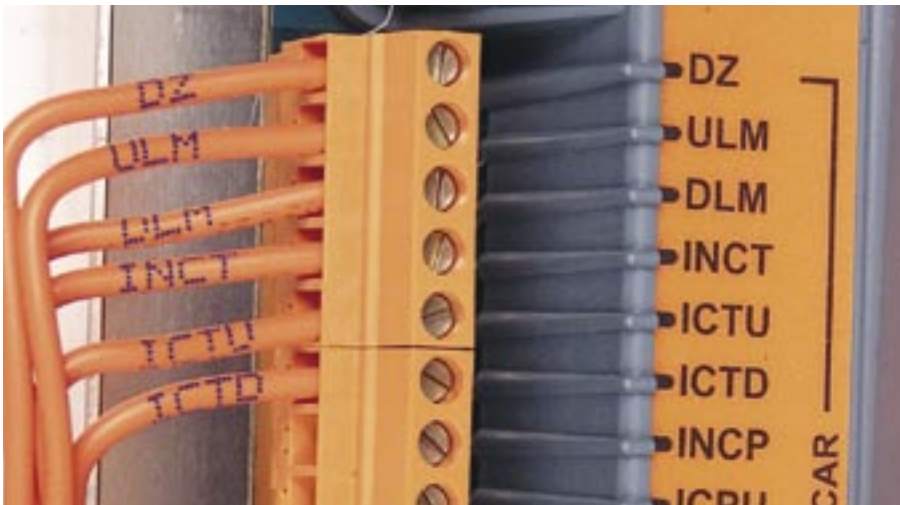
Typical label stamping at controller end
